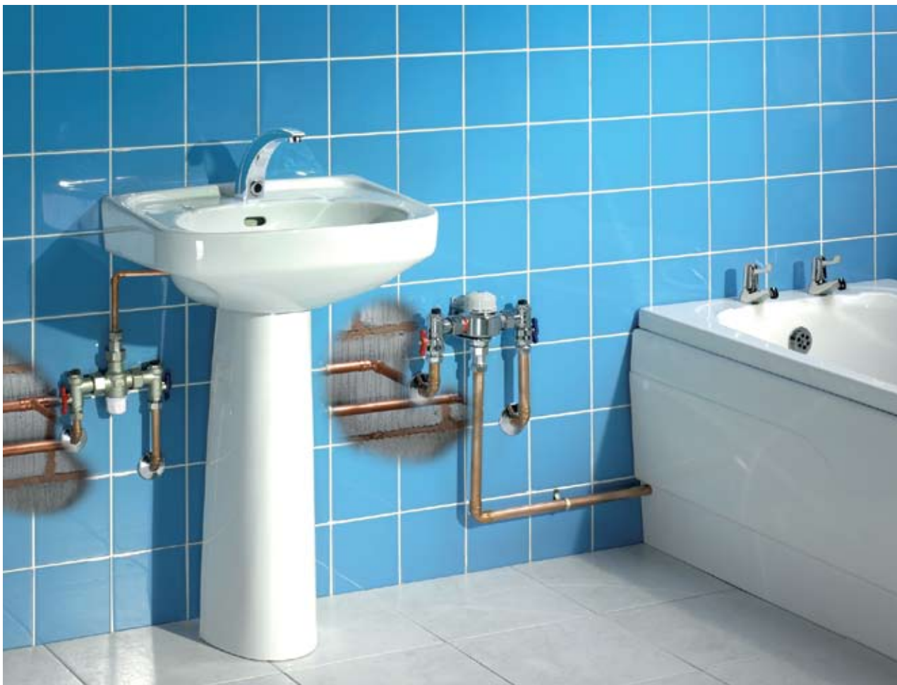
A typical installation, showing a Heatguard TMV3-8 valve fitted to control the hot water temperature at a handbasin and Promix 22-2 fitted to the bath supply.
